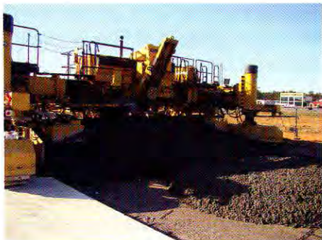
A Gomaco 2800 paver places concrete, with dowels and baskets in place, at a rate of 1800 cubic yards of concrete per day.
